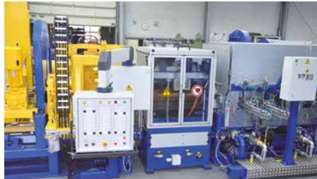
This photo shows an IAS induction heater installed directly after the extrutec gas heater in patented 'in-line' configuration during workshop assembly.
