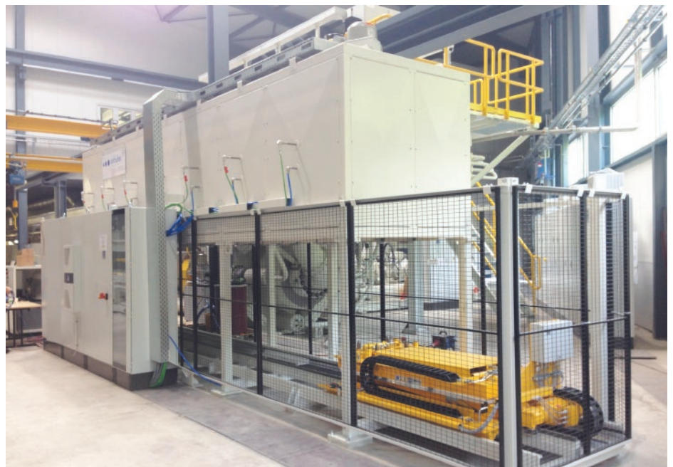
Die heating system installed at Aluminium Laufen in Switzerland.
